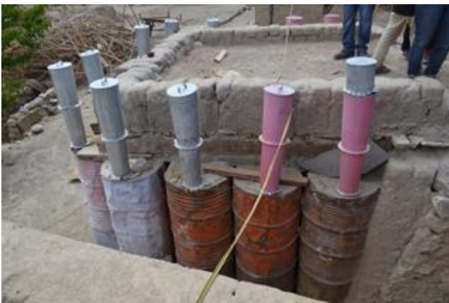
Underground Storage Units at SECMOL
