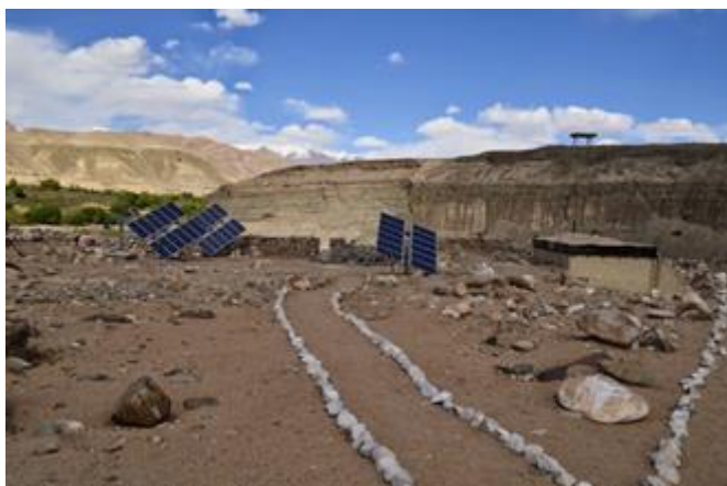
Solar panels which charge batteries SECMOL
